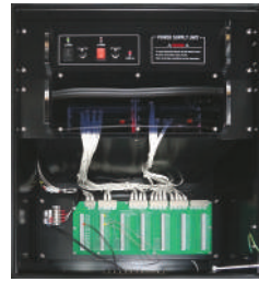
SME-144D (Telephone Exchanger)
